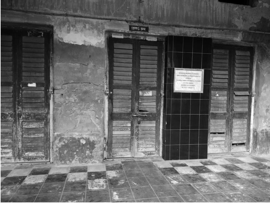
FIGURE 11. The shuttered Record Room of the Naogaon Ganja Cultivators' Co-operative Society in 2017. Water damage, infestation, and crumbling paint have destroyed much of the Society's archives. The plaque reads: "The Office Building of the Naogaon Ganja Cultivators' Co-operative Society Ltd. Opened by the Hon'ble Nawab Syed Nawab Ali Chowdhury, C.I.E. Khan Bahadur, Minister, Govt. of Bengal, on the 16th February 1921." Photograph by author.
